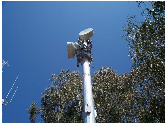
Emergency Communications Microwave Antennae at Eagle Rock
